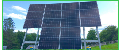
Vermont, USA Residential off-grid Homeowner in VT gains energy independence from the grid
